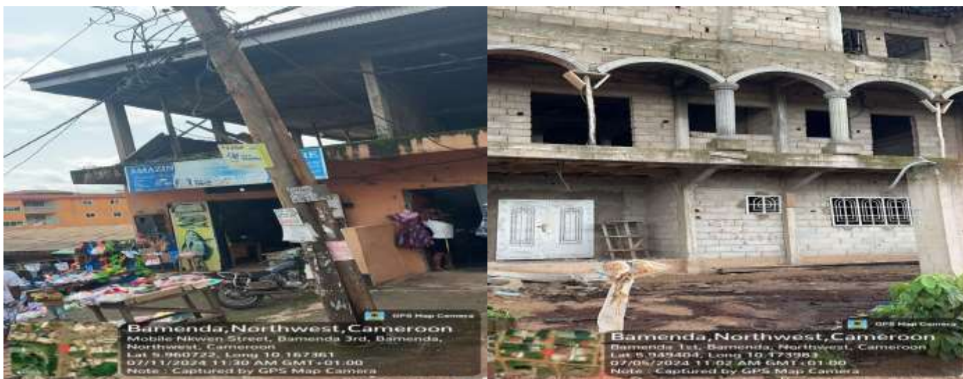
Figure 11: Housing with Poor Structural Quality
