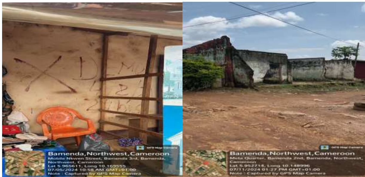
Figure 7: Aftermath of Housing Demolition Cause by Tenure Insecurity Issues
